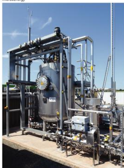
FIGURE 3. This biomethanation unit in Allendorf, Germany, uses microbes to convert hydrogen and CO 2 into methane
